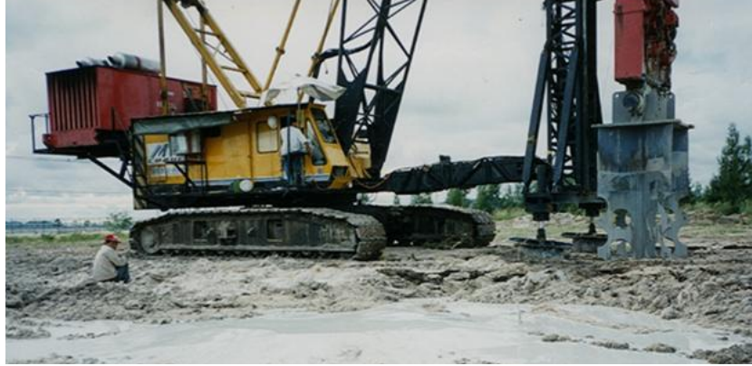
Fig. 10.16. Liquefaction of water-saturated sand during the initial phase of compaction. Note that water has collected on the ground surface. The original groundwater table was 4.5 m below the ground surface.
