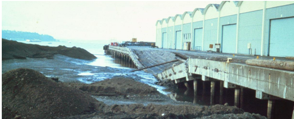
Fig. 7.51 View of the consequence of a hydraulic fill of fine silt flowing against 24-inch piles.
