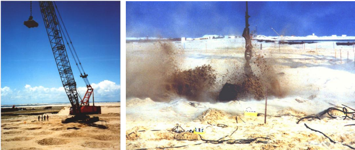
a) Compaction with 25 tonne mass and 25 m drop b) Vibration monitoring on ground
