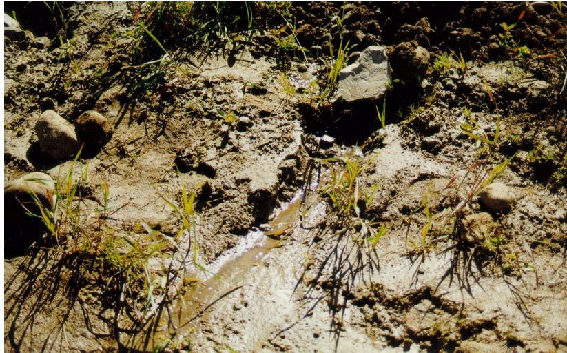
Fig. 4.10 Water discharging from a drain immediately outside the embankment
