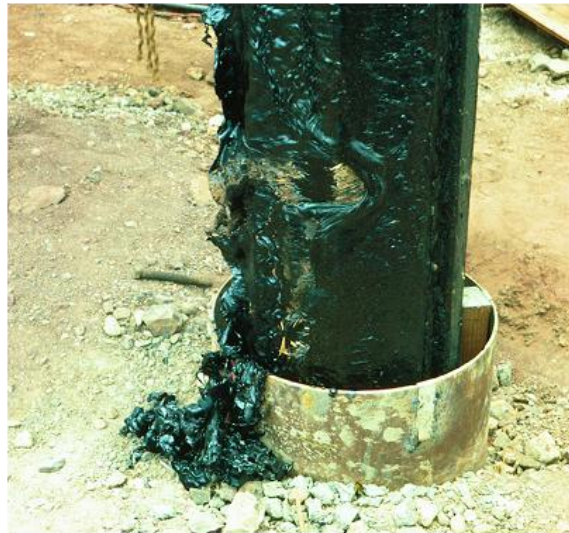
Fig. 7.50 View of a bitumen-coated pile driven through a protective casing The left side of the pile was the pile underside in storage
