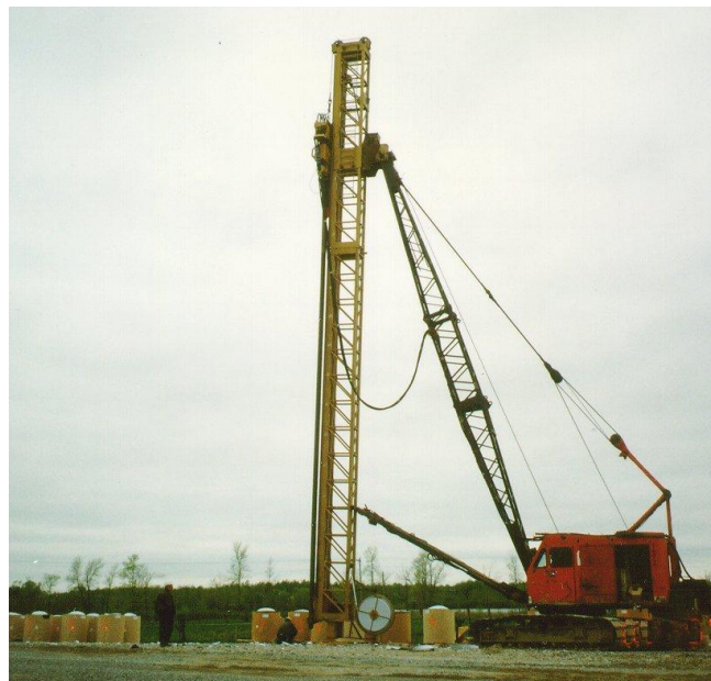
Fig. 4.11 Installation of wick drains type Alidrain (courtesy of J.C. Brodeur, Burcan Industries Ltd.)
